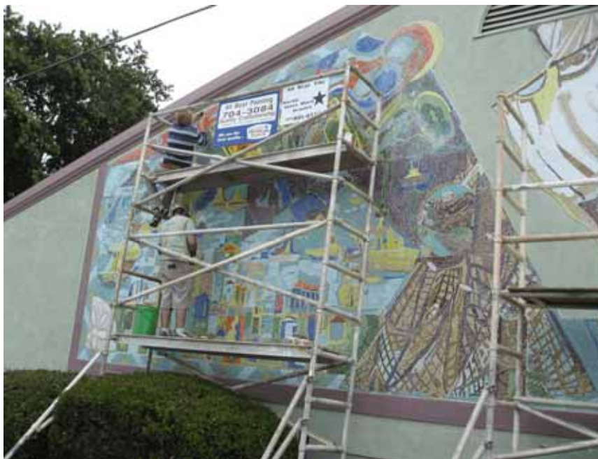
Ben Koppl working on the high board, while Steve Proano, master tile-setter, gets ready to replace missing tiles on the bottom level of the scaffolding.
